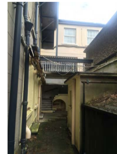
North (rear) wall of St. Teresa's - with structures at 1.2m and 3.2 m from facade
